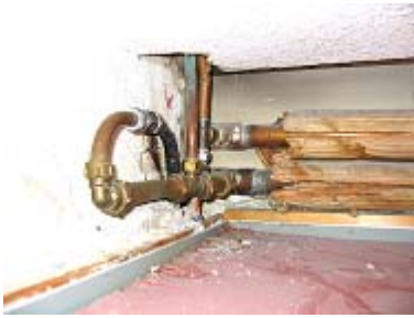
Figure 5: Example of poor insulation of circulation tubes.
