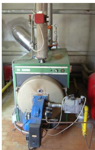
Figure 7: Forced draught boiler
