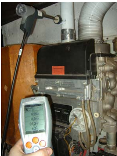
Figure 5: Boiler inspection. Basic boiler setting may be checked with a simple flue gas analysis. A check of the set maximum power can also give useful information.
